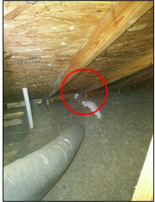
Not vented to exterior
