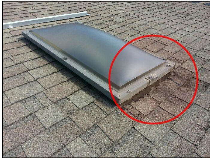
Wrong, incomplete flashings
