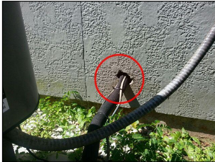
Caulking missing or ineffective
