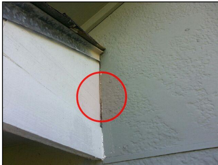
Caulking missing or ineffective
