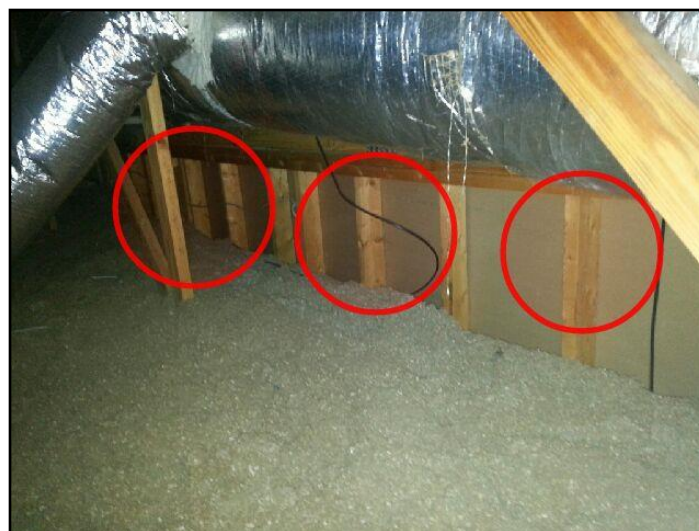
Missing at dropped ceilings
