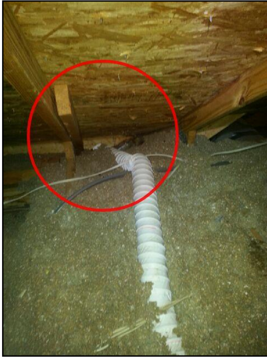
Not vented to exterior
