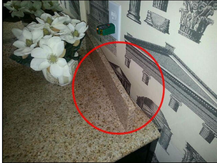
Loose or missing pieces
